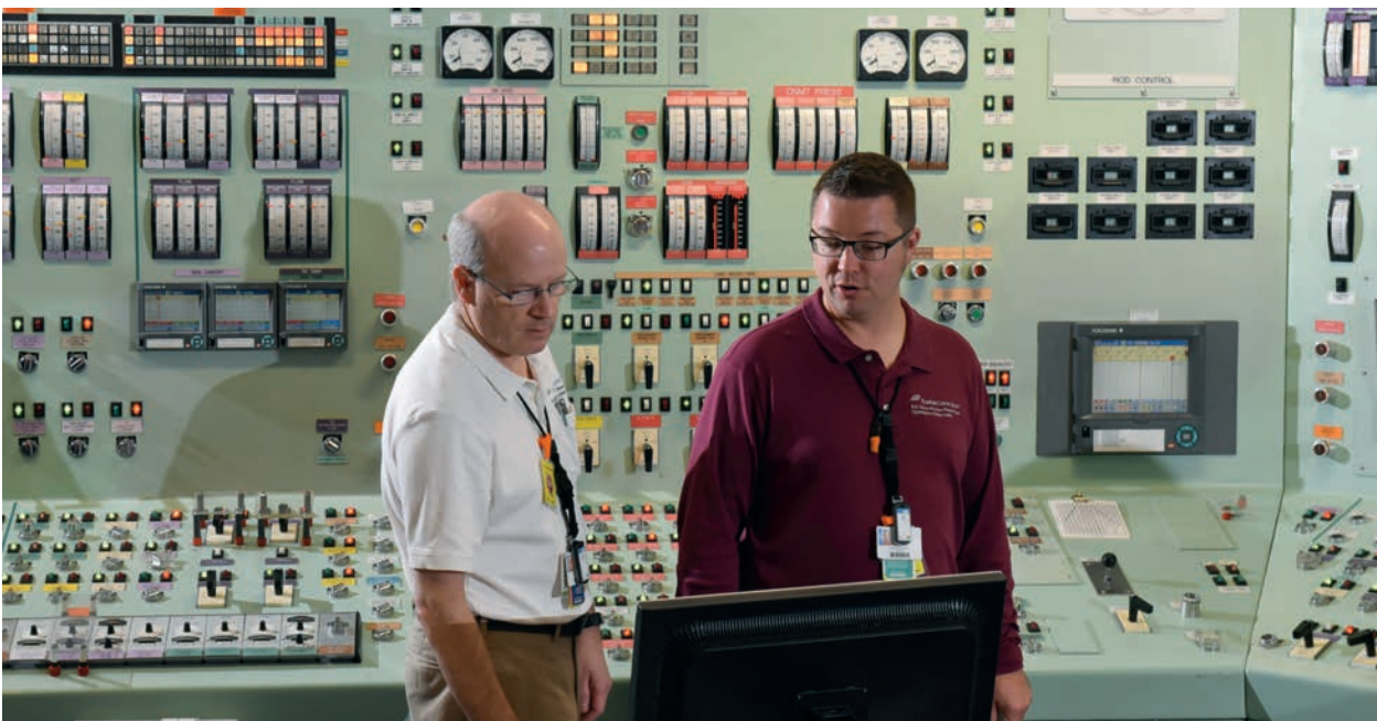
Control panel of R.E. Ginna (Image: Exelon)
